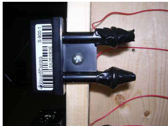
Figure 33: Terminals with electrical tape
