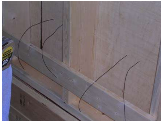
Figure 4: Plywood Layer sensor wires, rear view
