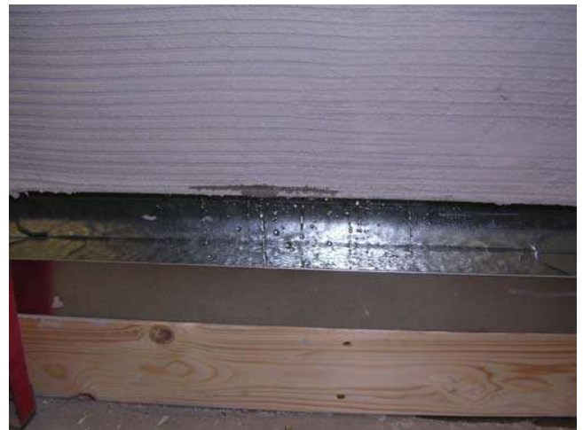
Water dripping into collection pan
