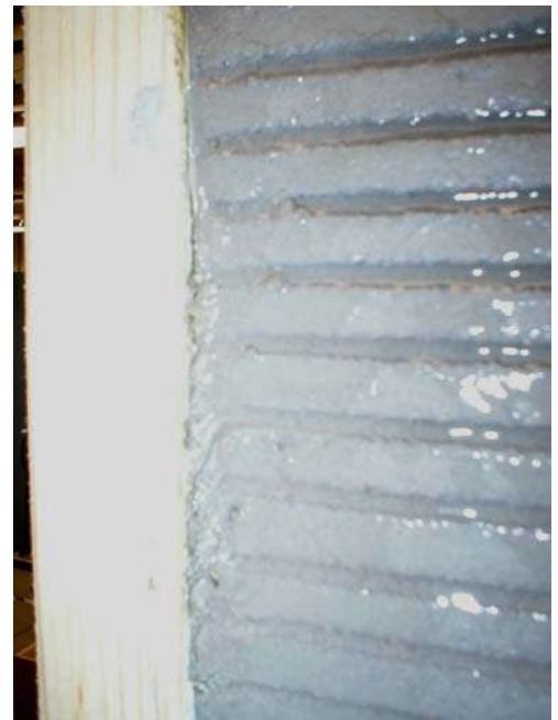
Water running along outside edge of Wall A on first test
