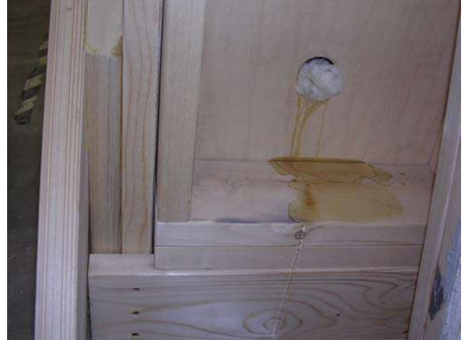
Water running from back weep hole of Wall A
