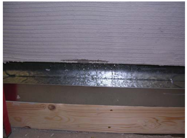
Water dripping into collection pan
