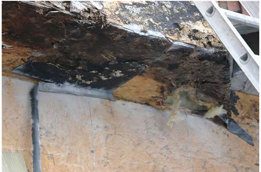
Figure 2: A “stucco bucket” on this stuccoed cantilever resulted in the wall kicking the bucket, so to speak. Water had nowhere to drain and eventually overwhelmed the WRB, rotting the framing beneath.
