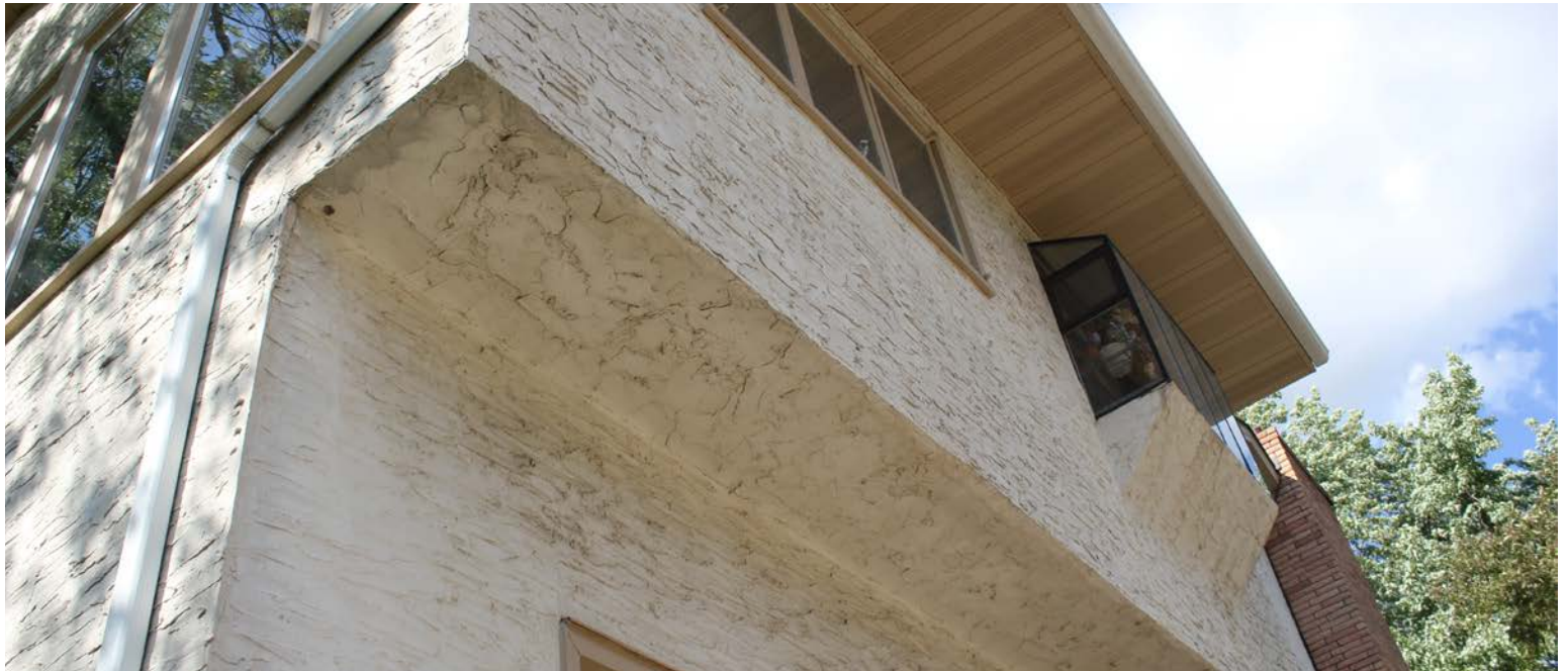
Figure 1: When stucco changes planes without a plan for drainage you get a stucco bucket. Buckets hold water - stucco wrapped soffits will too.
